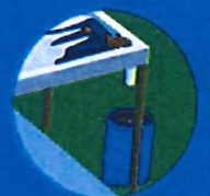
Flat roof without adequate drainage
